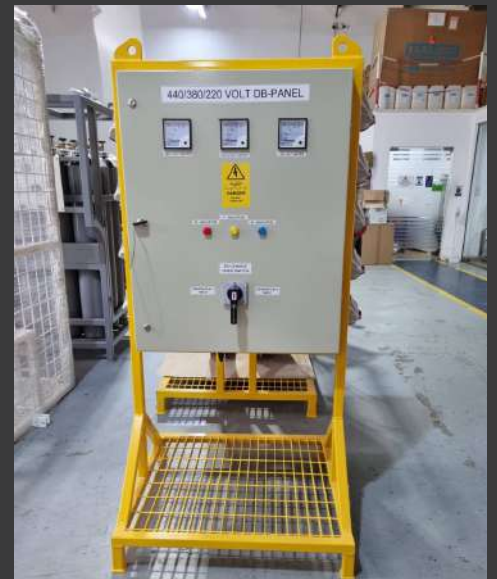
Electrical portable distribution board
